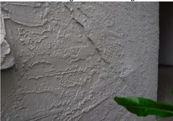
7 Area of Damaged Stucco Cladding
