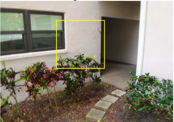
5 Area of Damaged Stucco Cladding
