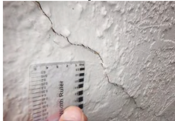
6 Area of Damaged Stucco Cladding
